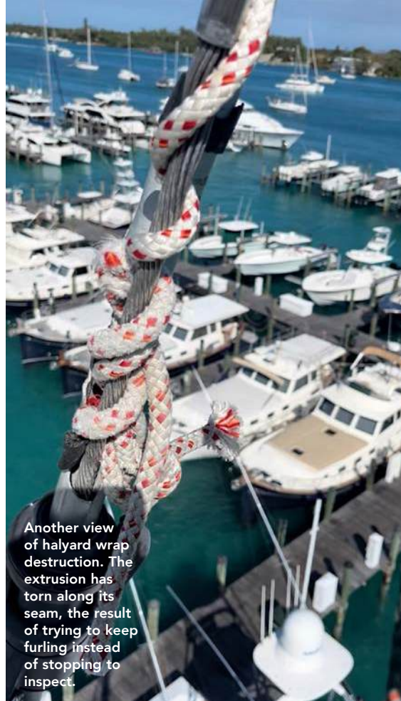
Severe structural failure from repeated halyard wrap. The foil has split completely, showing how easily a small lead-angle error can destroy a furler.
